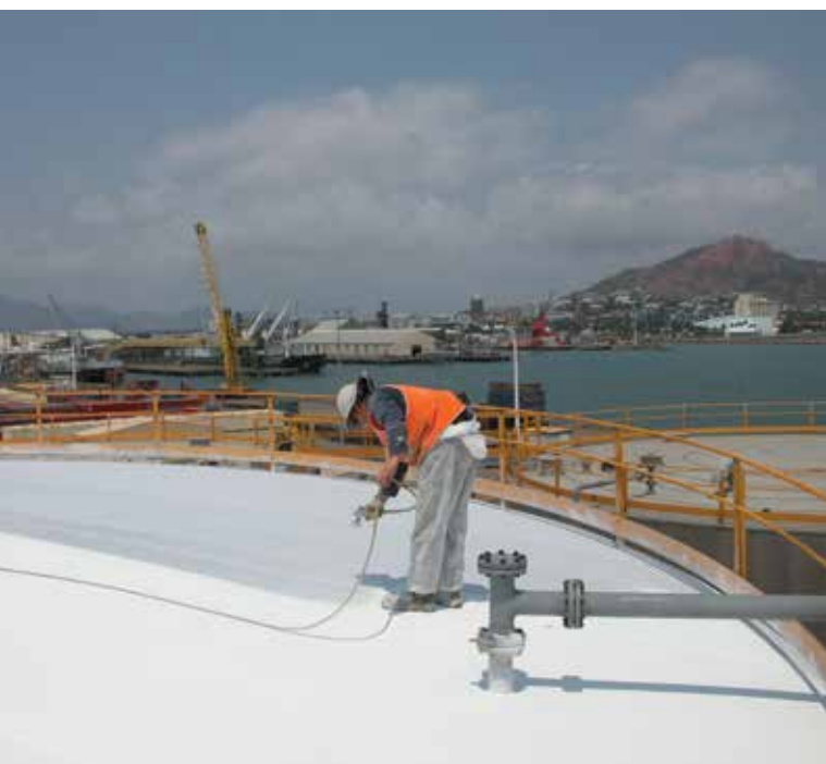
TICs are able to be applied quickly by as few as two to four workers on large areas, and allow foot traffic after installation
