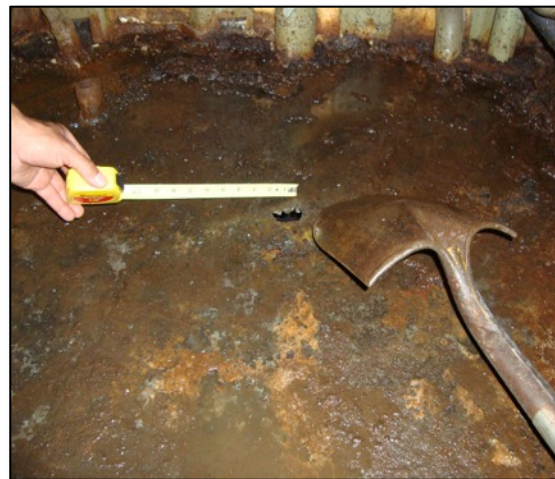
Floating floor after CUI
