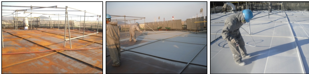
Corrosion was sandblasted, followed by priming, and then Mascoat Industrial-DTI was applied.
