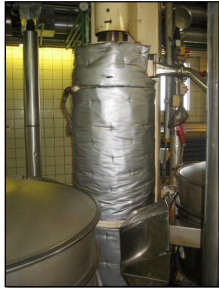
Traditional insulation that became flammable after absorbing grease.
